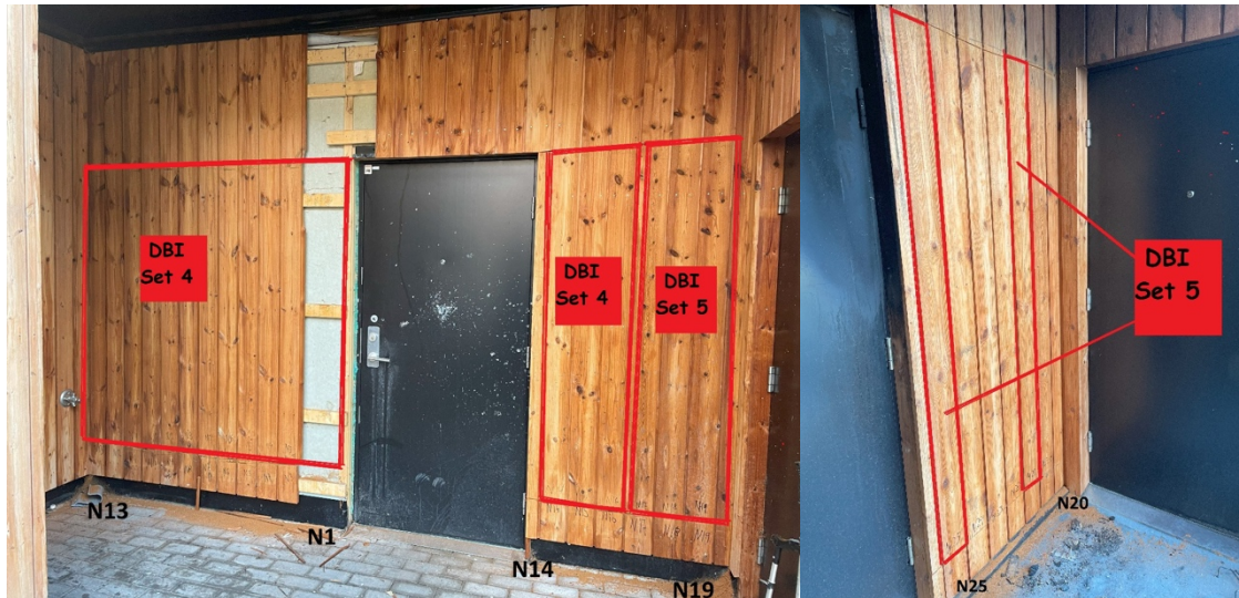
Figure 4: "Protected" boards from the north side of the building. The pictures show what samples that were taken for testing at DBI.
