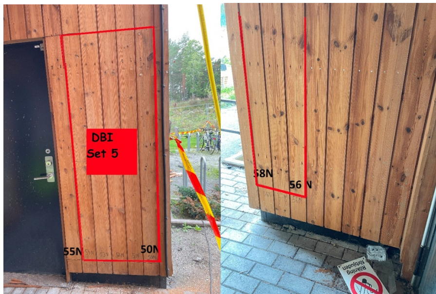
Figure 5: "Protected" boards from the north side of the building. The pictures show what samples that were taken for testing at DBI.
