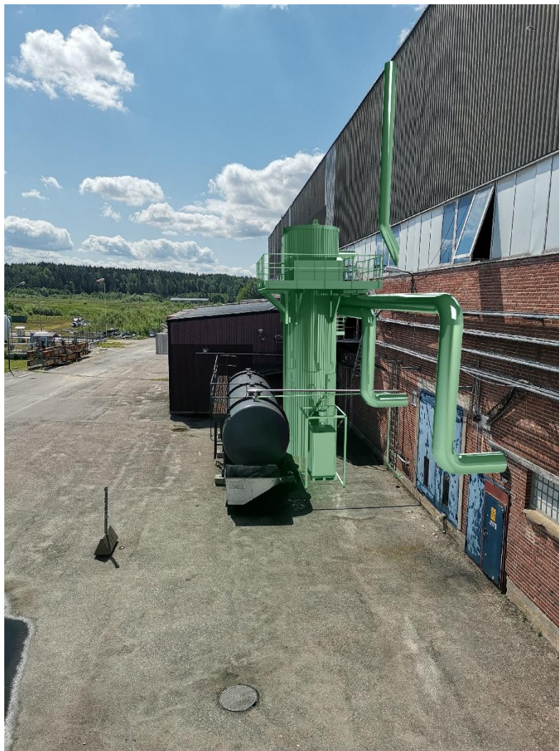
Above: This shows a layout of how an improvement of our flue-gas cleaning will look in our plant in Åsensbruk
