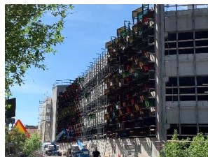
Installation is underway of the colorful solar cell modules for the garage in Mölnlycke Fabriker.
