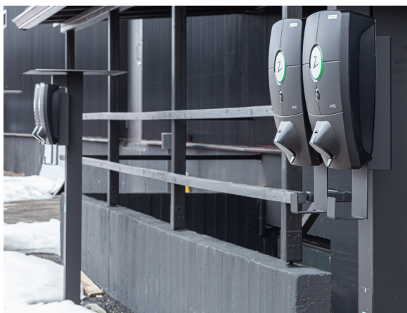
Installation of the electric vehicle charging stations at Ruosilantie 14 in Finland, which also has an ongoing BREEAM In-Use sustainability rating.
