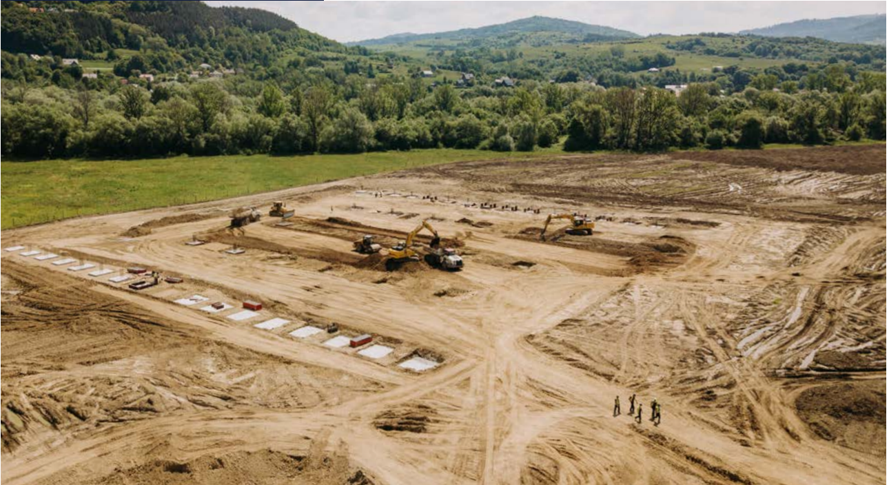
In May, Bulten started the construction of a new manufacturing facility in Radziechowy-Wieprz in Poland.
