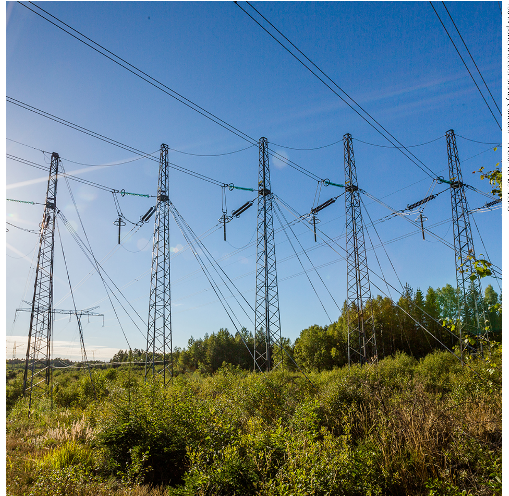
400 kV power line Letsti-Svartbyn, Sweden | Photo: Tomas Arlemo
