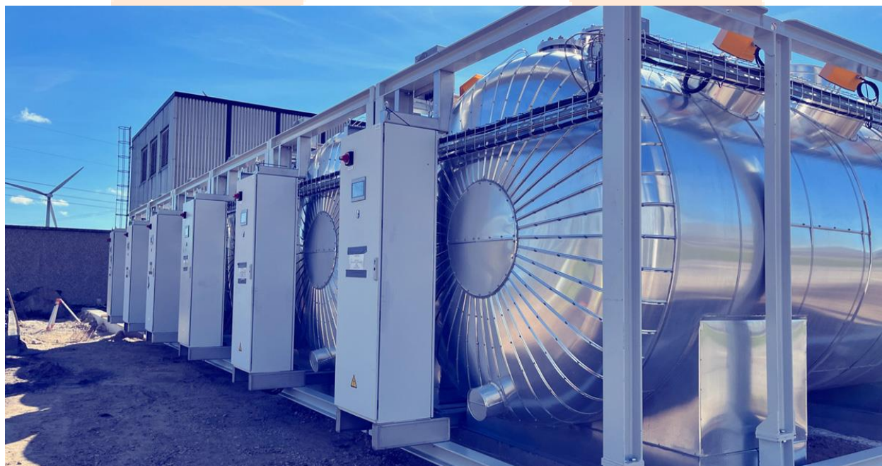
CAPTION: Commissioning of Norbis Park Heatcube
