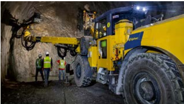
The work on the 125-kilometer Rishikesh-Karnaprayag Railway Line in the Himalayas is in full swing. The greenfield project has a total tunneling length of 218 kilometers. Here, Epiroc's automated and semi-automated machines, incl. the Boomer E2, are being used and contribute to increased efficiency on-site and reduced cycle time.
