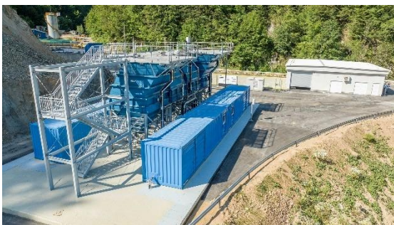
Image: Modular treatment plant for mining water at Ellatzite-Med in Bulgaria
