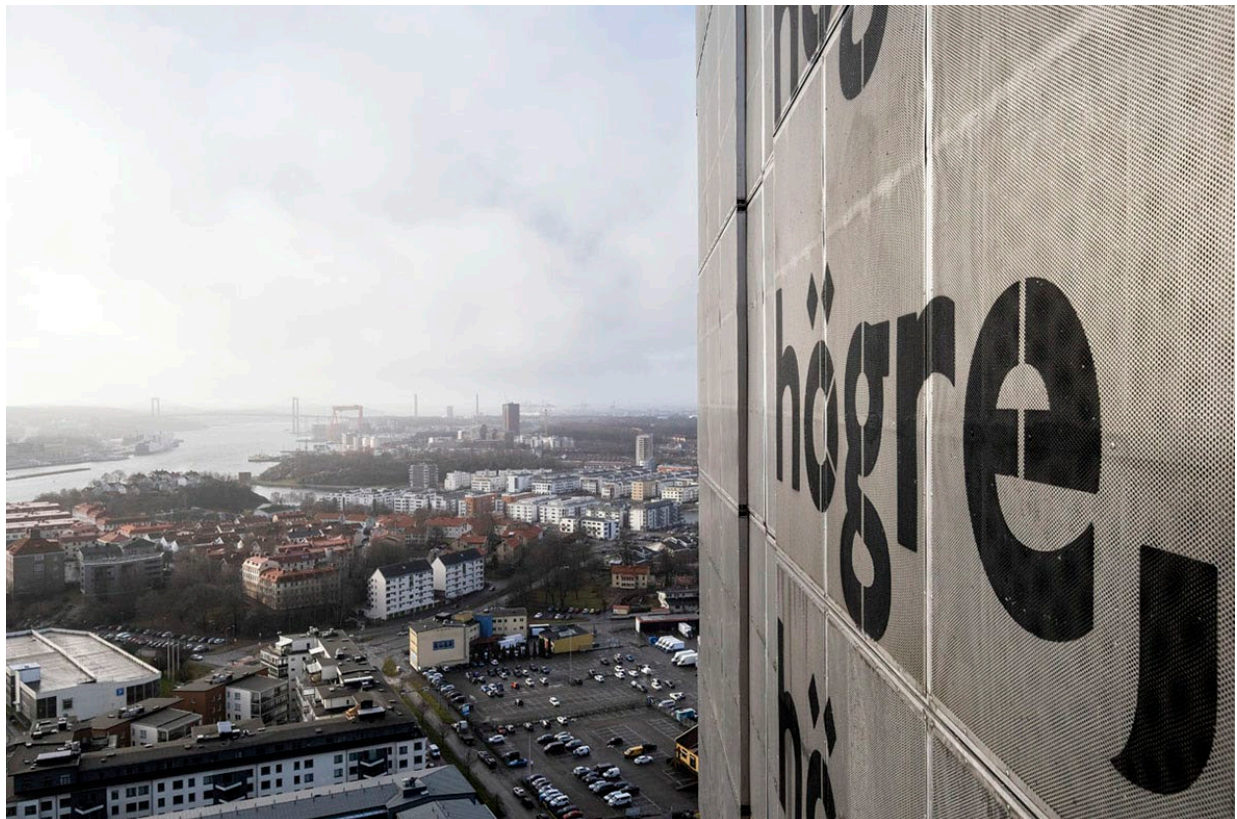
At the end of 2021, Karlatornet passed one hundred meters in height and continues to grow by about one floor a week. Photo: Kasper Dudzik
