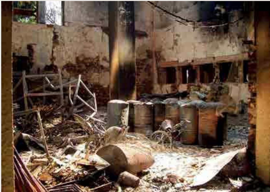
A view of the damage after the attacks by the Lord's Resistance Army (LRA) rebels on the central store at the Nagero airstrip, north-eastern Democratic Republic of Congo. REUTERS/Stephane Carre, 2009.
