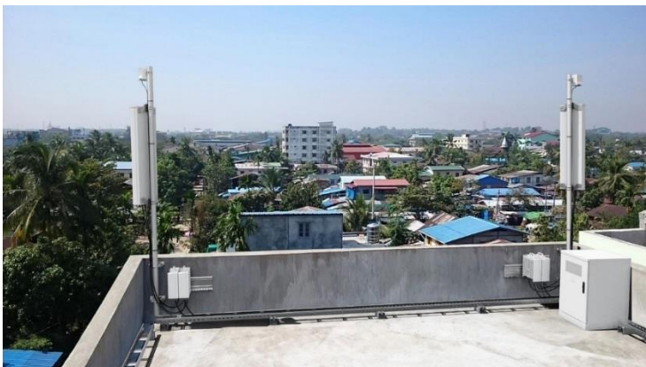
Ericsson radio site solution for developing markets, including newly launched Radio 2219, GSM + WCDMA, rail mounted on the wall, MINI-LINK 6363 and Enclosure 6130.
