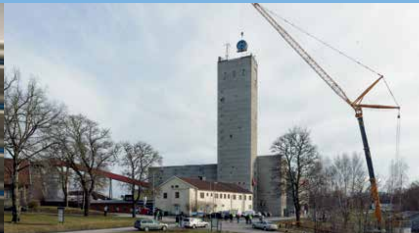
The 19-tonne winding drum is installed at the top of the head frame, which is 78 metres high.
