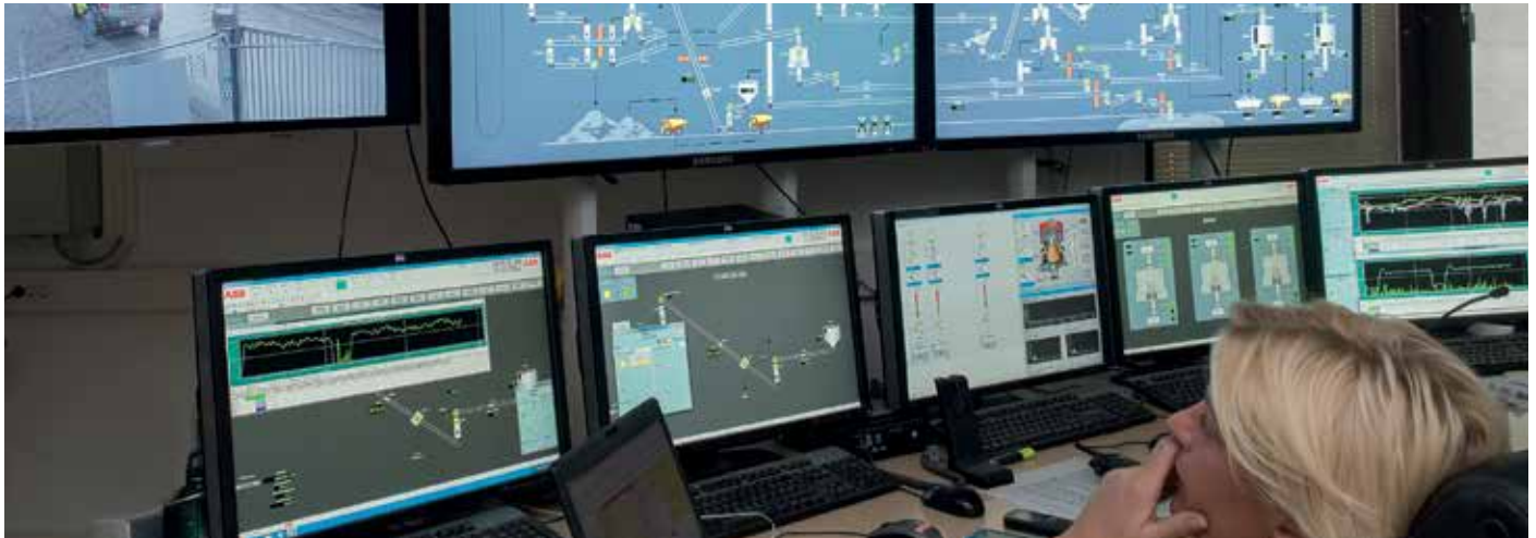
Production at the sorting plant is monitored and controlled from the control room, which is housed in the renovated office building.
