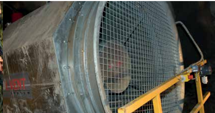
The installation of the mine's ventilation system is in progress. Completion in 2013.
